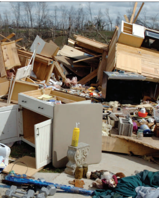
An ill wind: an April storm destroyed this house in Tennessee, and the weather seems set to worsen.
