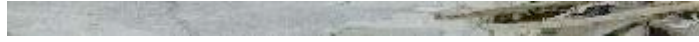
In Pensacola, Florida debris from demolition and rebuilding after Hurricane Ivan last year. (Photo by Andrea Booher courtesy FEMA)
